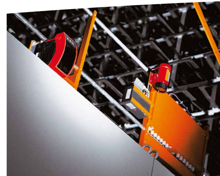
Optical data transceiver and laser axis ensure safe data transfer and trouble-free positioning of the operating gantry crane.
